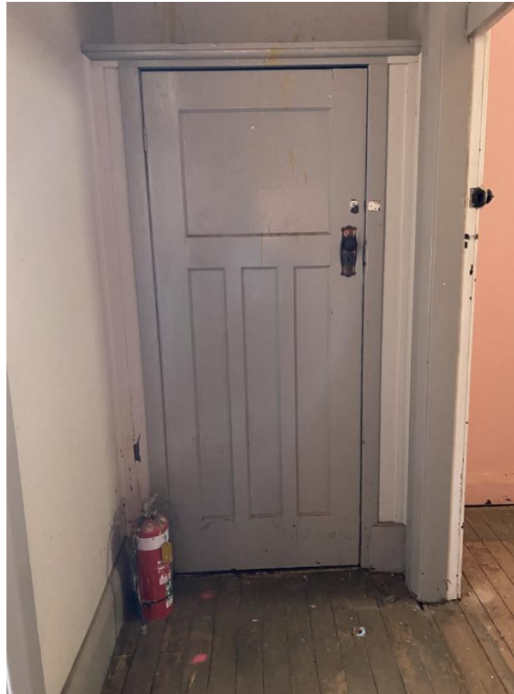
Figure 6.4.2 Extinguisher not mounted on wall and not in a compliant location.
