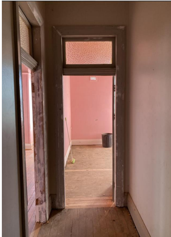
Figure 6.2.5 Infilled fan light not achieving an FRL above the doorway to an SOU along with a doorset that does not comply with C3D12
