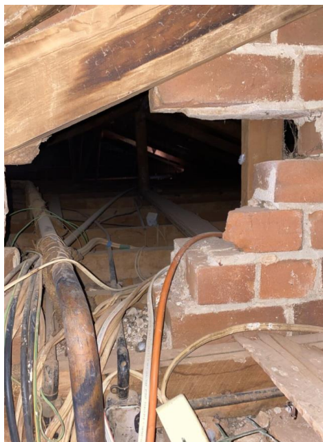
Figure 6.2.6 Observed onsite a hole where services pass through a bounding wall within the roof cavity
