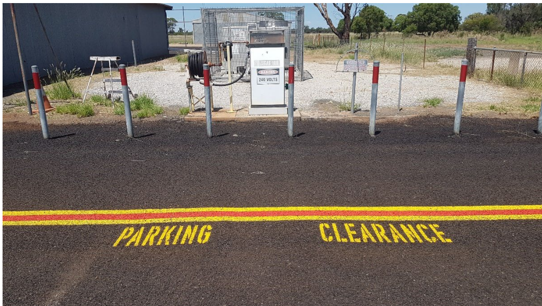
Figure 2 Condobolin Airport fuel facility
